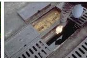
Perimeter Sand Filter
