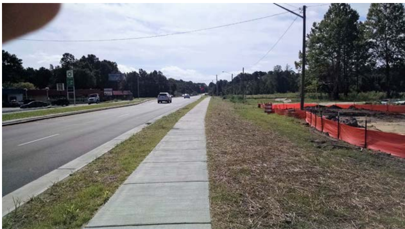
New sidewalk construction costs vary on several factors. Further design is needed to develop detailed project costs.
