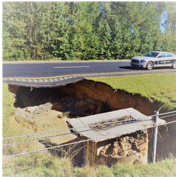
FIGURE 5.12: SINKHOLE IN NORTH CAROLINA
